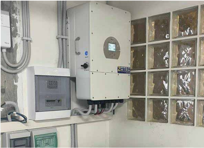
Italy ▶ Inverter: SUN-6K-SG Capacity: 6kW
